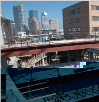
Expansion project: Walkways on the fifth and sixth floors and on the roof extend over the building's open courtyard. Located on the fourth floor, the courtyard will provide a quiet place of reflection for patients and visitors.
